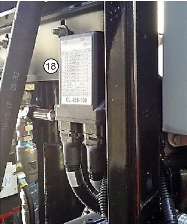
Figure 5-9: Recycling I/O Module at Back of Cab
