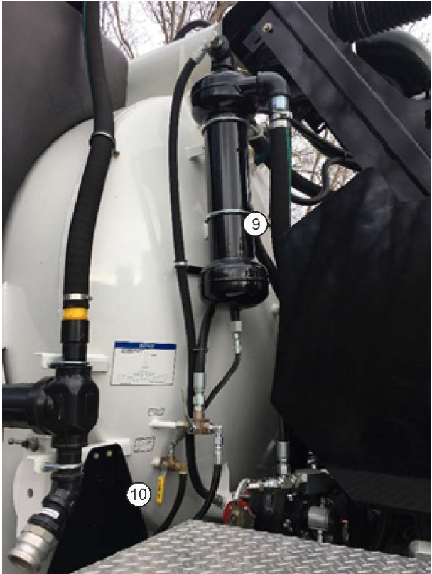
Figure 5-4: Cyclone Separator and Drain Valve
