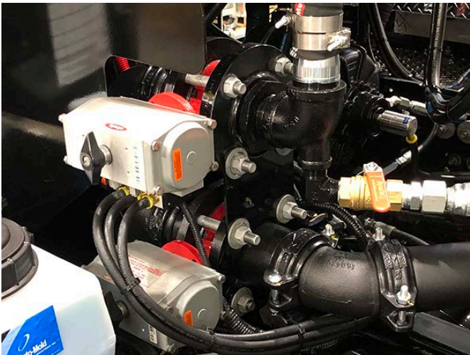
Figure 5-5: Water Supply Valves
