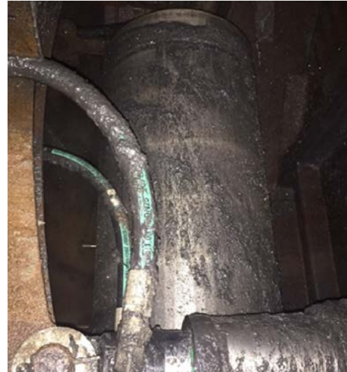
Figure 5-37: Tank Filter Clogged with Grease
