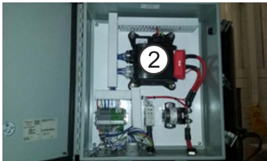
Fuse and Relay Box
