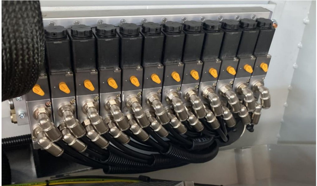
Figure 3.17: Pneumatic Control Panel
